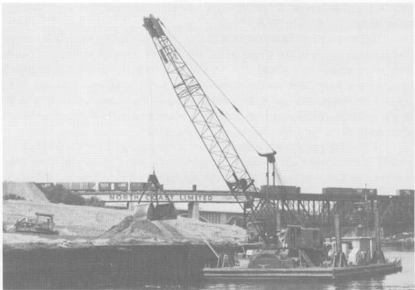
Stockpiling dredged material in St. Paul, Minnesota, for future use as fill for recreational or industrial land, for creation of marshes, or even for sanding icy city streets. St. Paul District
