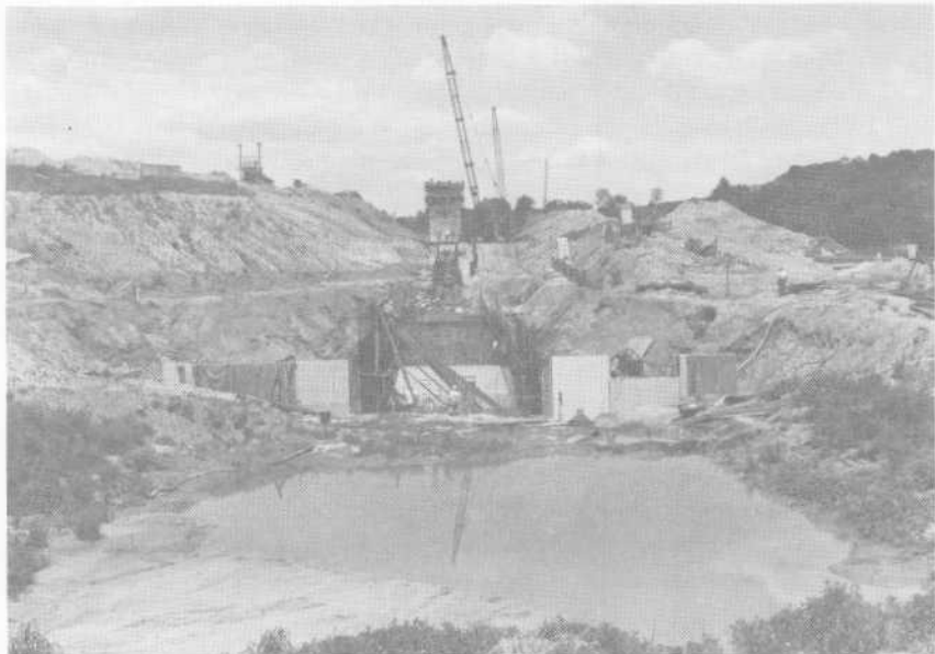
The La Farge lake and dam under construction in June 1973. The Corps stopped construction in April 1975 because of opposition from environmental groups and Wisconsin state officials.
